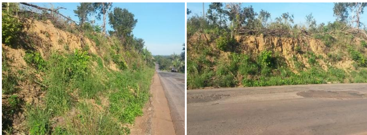
Foto 106 e 107: km 25,2 a km 24,78 – C=150,0 m, H= 4,0 m e L= 1,0 m.
